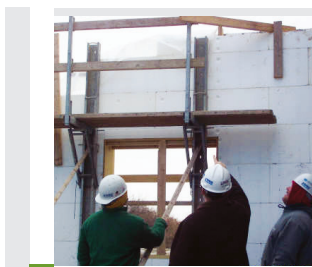
Locally deployed technical support staff
